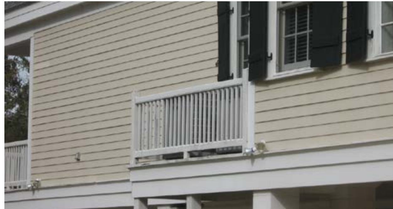
Elevated HVAC units should be screened from view with wooden or lattice panels.
