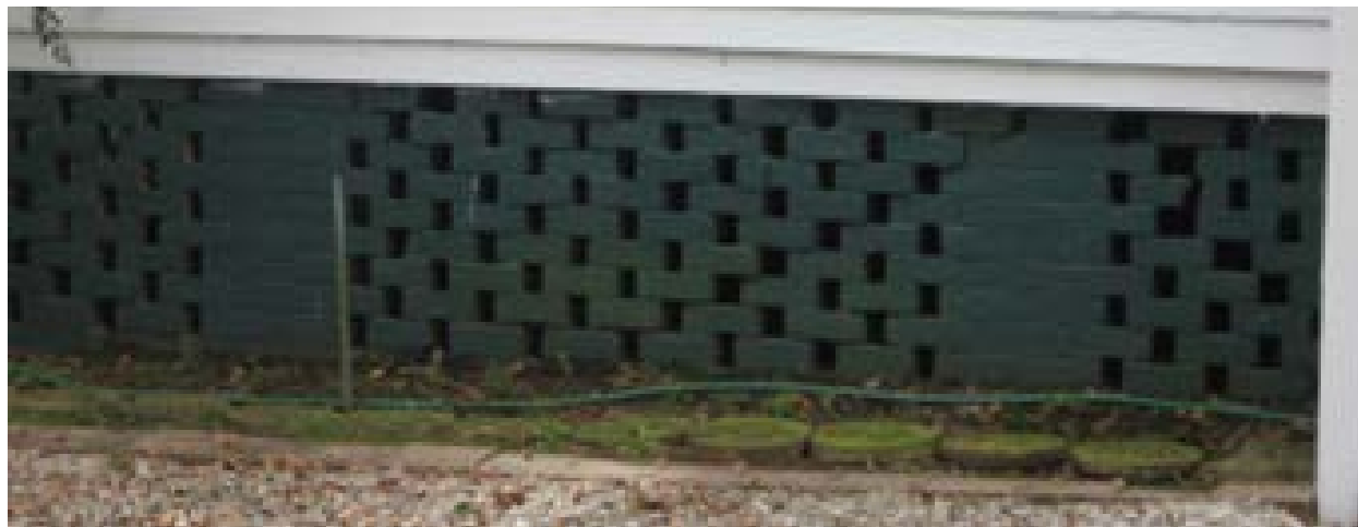
Historic vent patterns such as honeycomb brick should be preserved and retained (photograph above and below).
