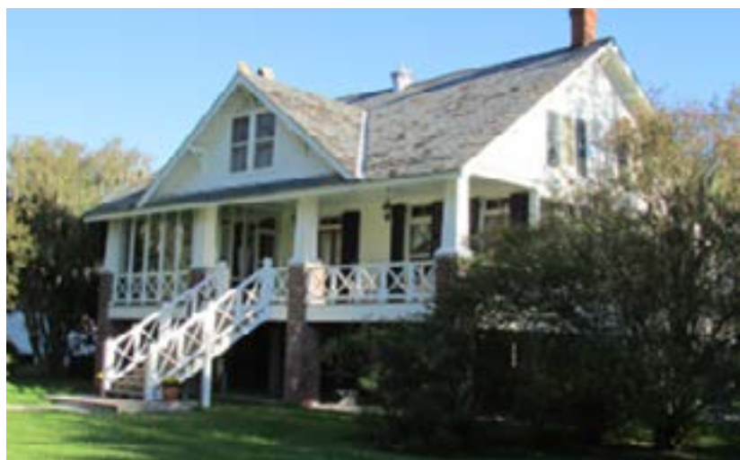
In a typical elevation project, a dwelling is lifted off its foundation and gradually raised with jacks and frame cribbing. Once the house reaches the Design Flood Elevation (DFE) it is placed on a newly constructed foundation. (Photos courtesy Rod Scott).
