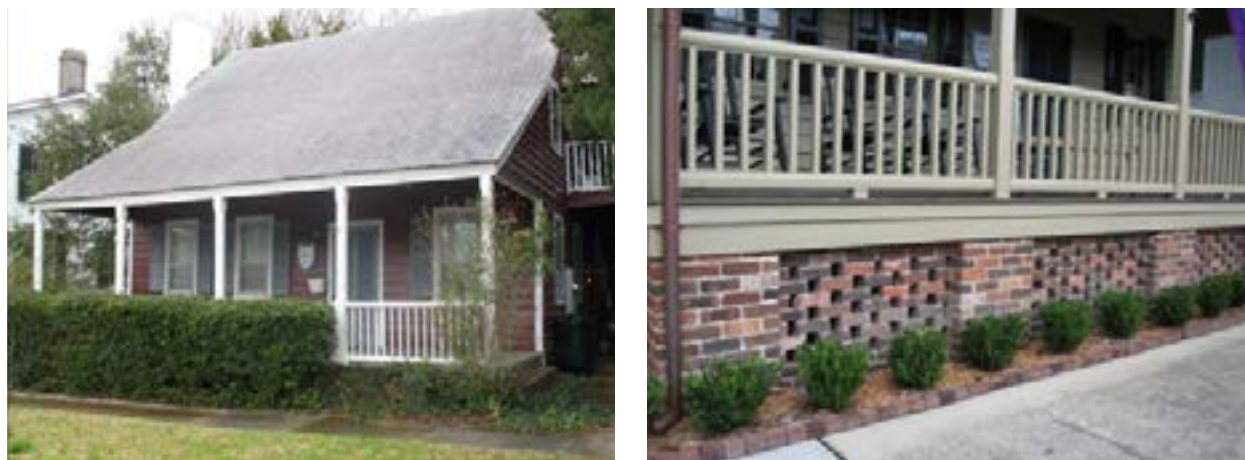
The elevation of this dwelling (above) included rebuilding the brick porch foundation with honeycomb openings for wet floodproofing (below). New flood vents meeting FEMA standards were added to other areas of the foundation.
