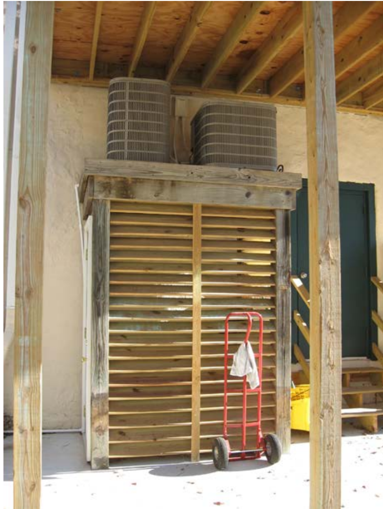
Utilities were removed from the basement of this historic commercial building and elevated on a rear platform beneath an added deck.
