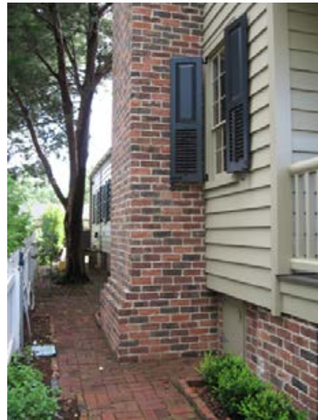
The elevation of this dwelling included rebuilding the base of the chimney with brick and mortar to match the original.
