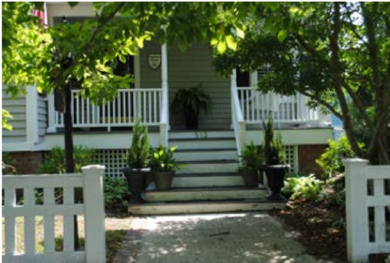
This building elevation project has added wide stairs below the original stairs to assist in keeping the stair railing at its original location and maintaining the porch design.
