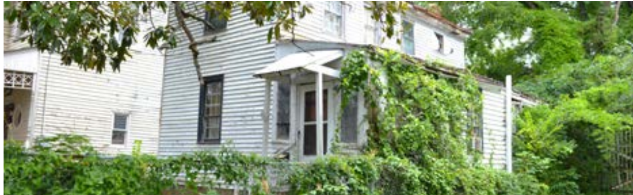
Deteriorated House 507 Ann Street
