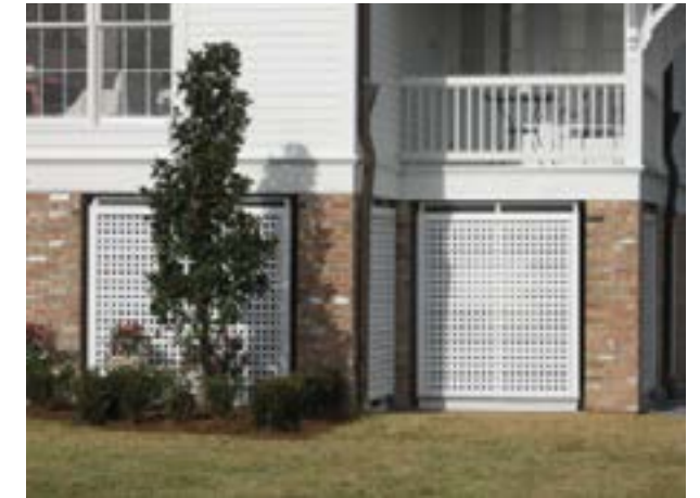
Break-away wood lattice panels are appropriately placed within the piers of this foundation.
