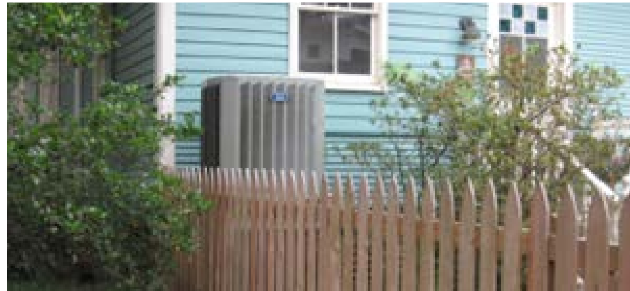
Site HVAC units on platforms at the rear or not readily visible side locations.
