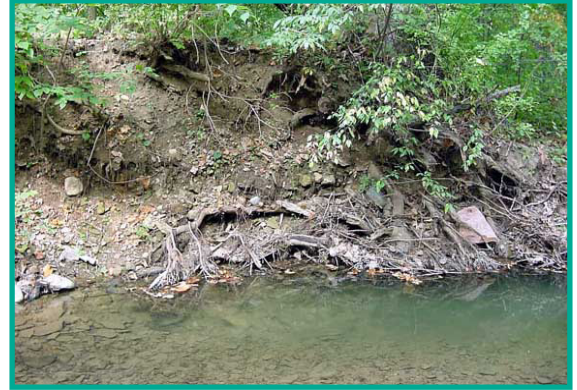
Sediment is washing into the creek and trees are falling into the water - a sure sign that the soil is unstable and the streambank is eroding.
