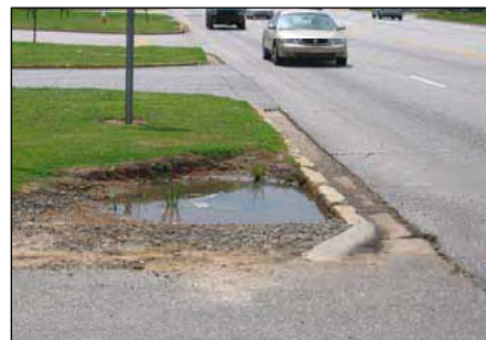
Damage due to insufficient curb radius
